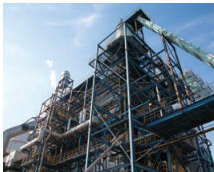
Gonoike Biomass Power Plant, Ibaraki
