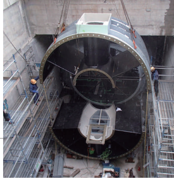
Shinkawa-kako Drainage Pump Station, Niigata
